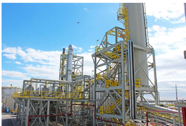
Figure 3. A 1 million tpy sulfur remelter with lime silo, external heat exchangers and a scrubber.
